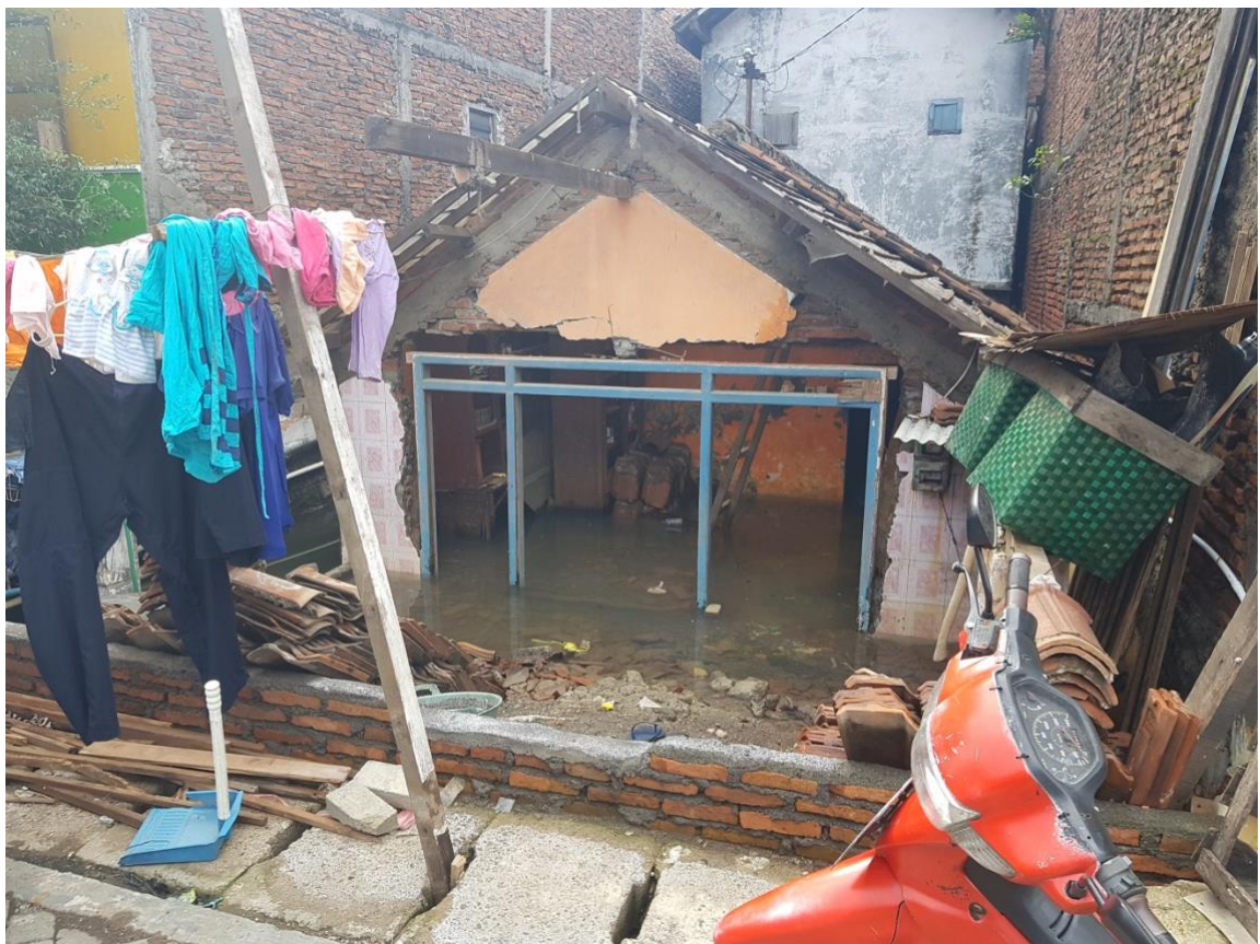
Figure 5: A flooded house in Tambak Lorok
