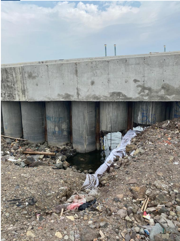
Breached coastal dike in need of maintenance
