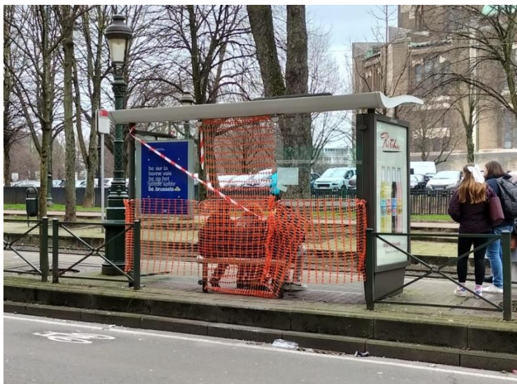
Figure 4.3.: Vandalized tram stop
