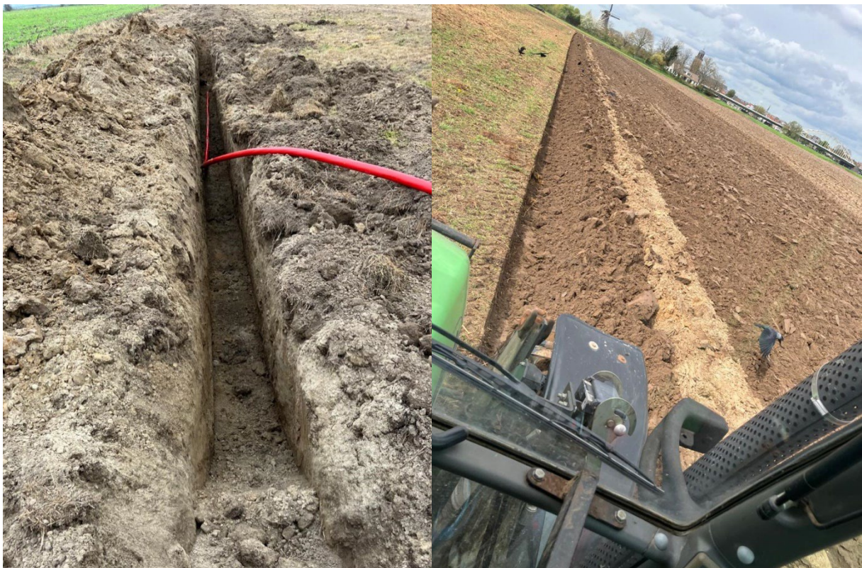
Figure 9 Example in which the different earth layers were not taken into account during the operation. Retrieved from the private collection of this senior advisor.
