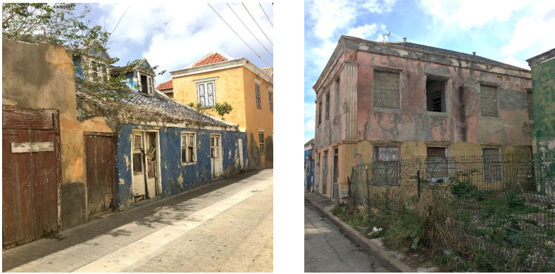
Figures 3.13 – Deteriorated and abandoned houses in Otrobanda (author, 07-06-2018)
