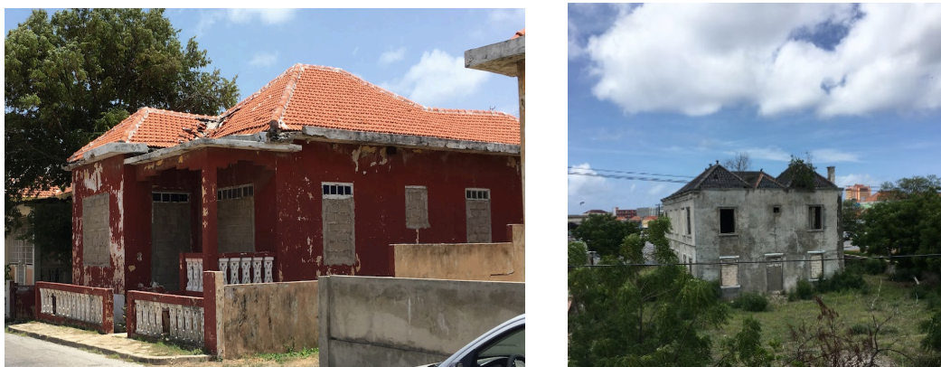
Figure 3.10 – Decay of houses in Scharloo area (Author, 2018)
