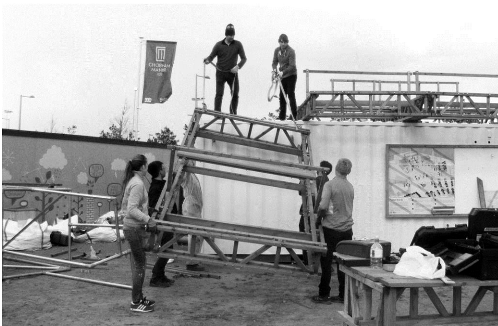
Figure 18. One difficult task: how to lift the roof structure on a container?
