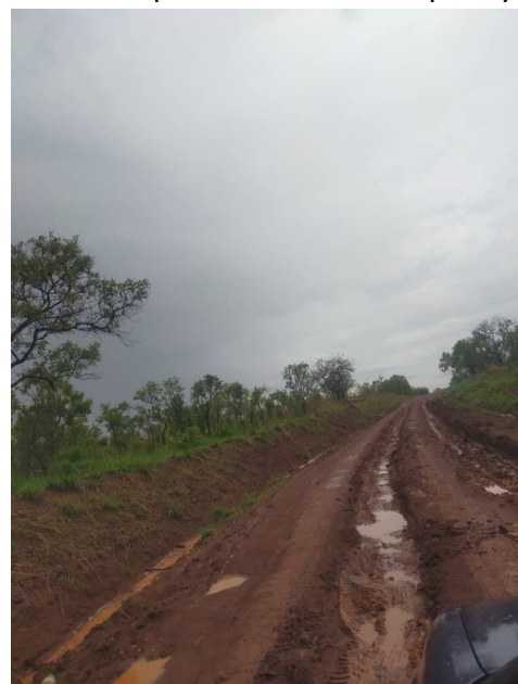
Figure 4 road after rainfall
