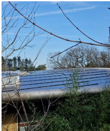
Figure 36 Solar panels Burgers' Zoo (1.1)
