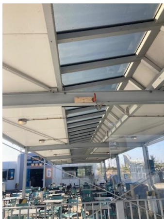
Figure 19 Solar panels WILDLANDS (2.5)
