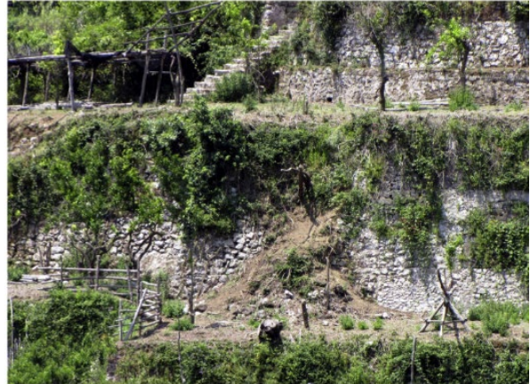
Figure 19, Terrace collapsing (Tarolli et al., 2014)
